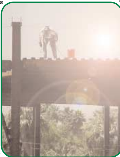
Unidentified worker conducting welding operations at a steel erection project in downtown Phoenix.
